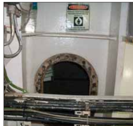
▲ This access is adequate but regrettably, the builders have put a cable run across the access
